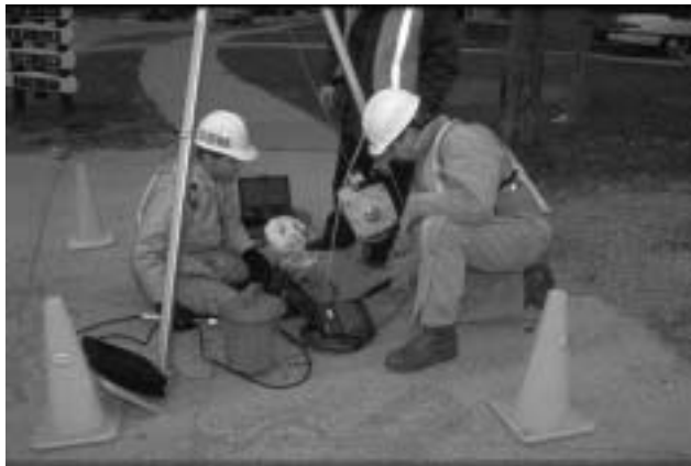
Ben Sherman and Mark TenBroek of CDM evaluate flow conditions in southwest Detroit as part of the Greater Detroit Regional Sewer System Combined Sewer Overflow (CSO) modeling work.
